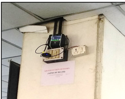
INDOOR UNIT AT FOYER AREA
