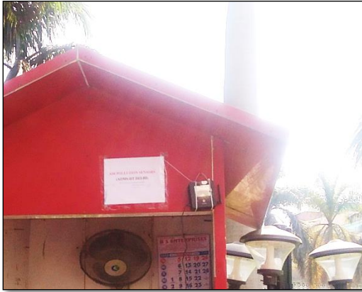
OUTDOOR UNIT AT GATE NO.2
