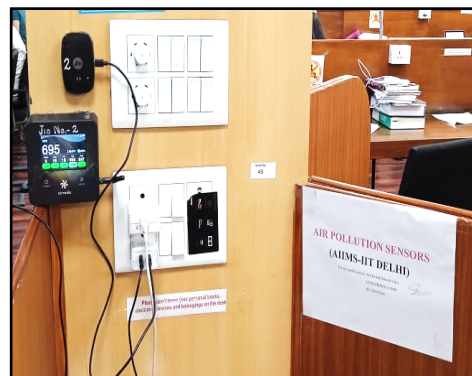
INDOOR UNIT AT B.B. DIKSHIT LIBRARY
