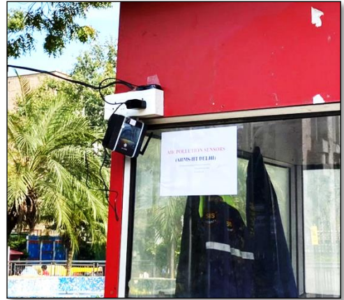
OUTDOOR UNIT AT EXIT GATE NO.1
