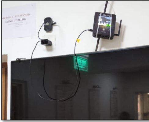
INDOOR UNIT AT OLD OT BLOCK
