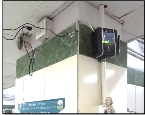
INDOOR UNIT AT MEDICINE WARD
